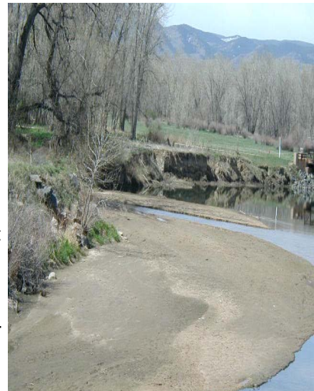
Eroded sediment can clog downstream receiving waters.
