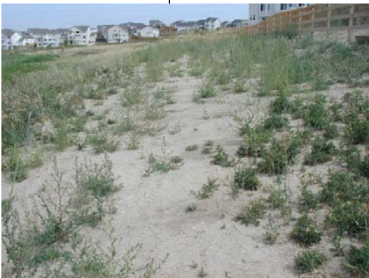
Common areas are often neglected during the construction of single family residential projects. Adequate perimeter controls were not installed at this site, resulting in sedimentation and weed infestation.
