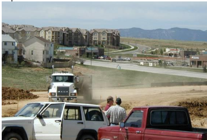
The GESC Manager shall always be available on site or by phone for communications with the County Inspector.
