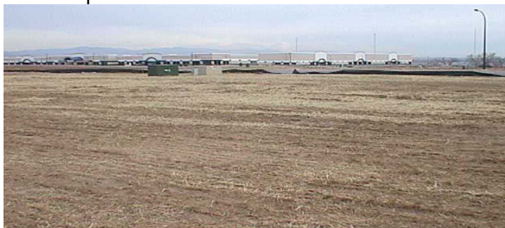
This site was issued a reinspection fee when the GESC Manager scheduled an inspection prior to reaching the required vegetative cover as well as not maintaining the required sediment controls.
