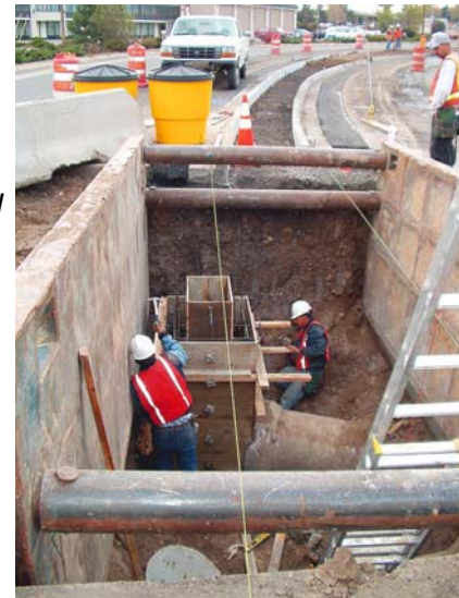
No utility trench shall be left open at the end of the work day.
